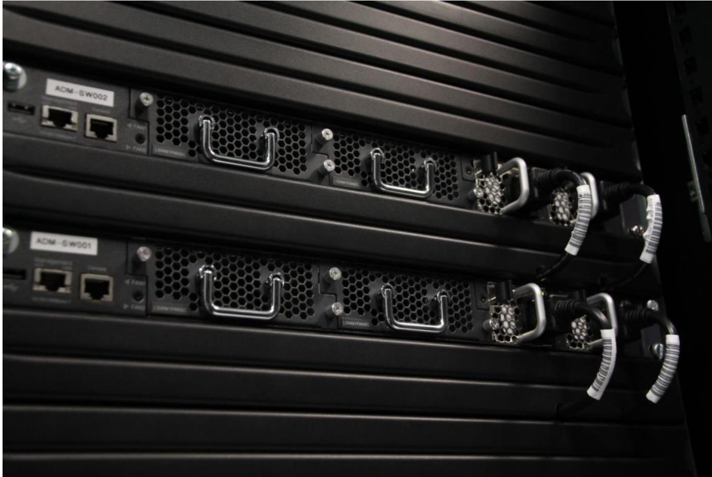
Redundant switches | redundant power | redundant cooling
