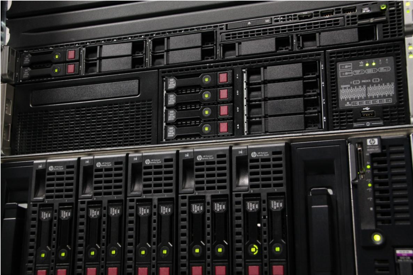
Redundant switches | redundant power | redundant cooling
